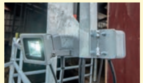
Power outlet and LED lighting
